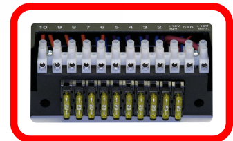
View of Terminal Block
